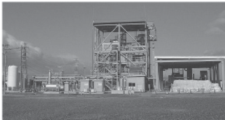
This large pilot biomass plant is in Japan
